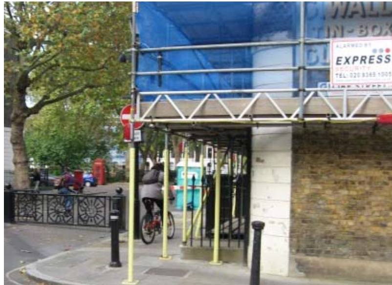
Figure 16: A cyclist using the footway of Trinity Street to bypass the carriageway barriers
